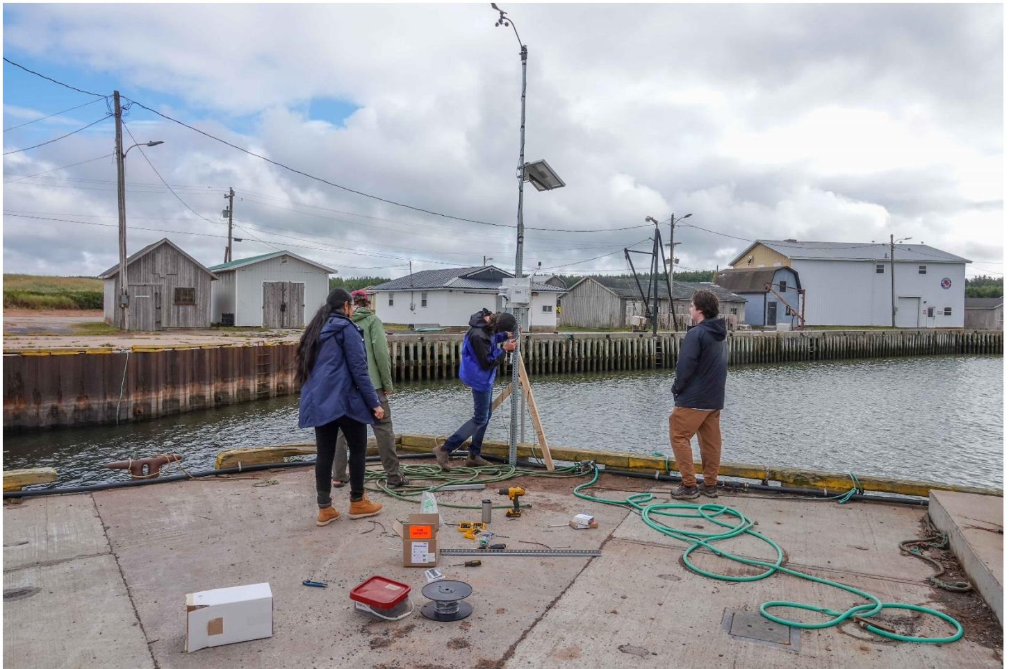
Figure 2: UPEI ACC-3030 Class Installing New Climate and Tidal Station at Naufrage Inner Harbour, Sept. 2022.
